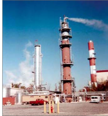
AES Warrior Run Power Plant Captures 10% of CO 2 from a 205 MWe (gross) CFB plant Cumberland, Maryland
