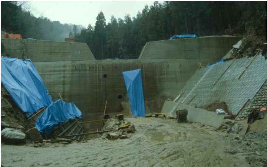
A large check dam just above the apex of a debris flow fan, near Hiroshima, Japan.
