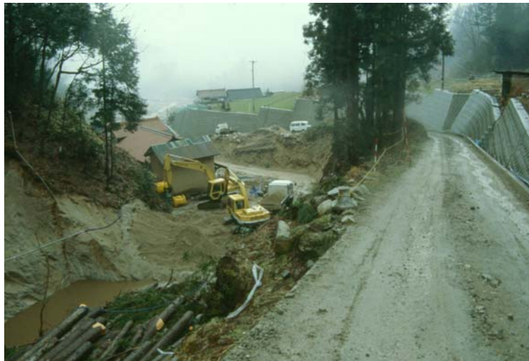
A debris flow deflecting dyke at the head of a debris flow fan near Hiroshima, Japan.
