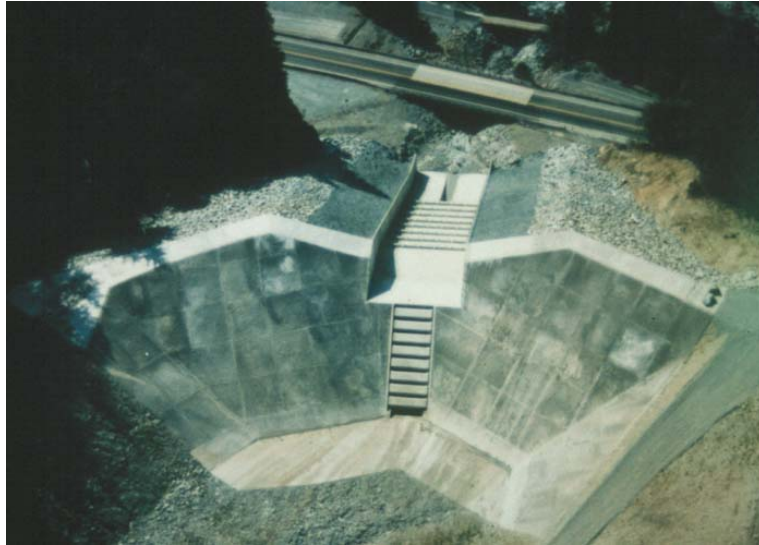
An engineered earthfill barrier on Charles Creek, Lions' Bay, B.C., designed to retain 30000 m 3 of debris
