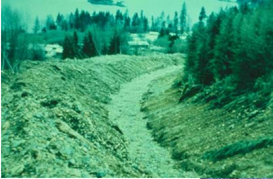
Deflecting dykes constructed around the community of Port Alice, Vancouver Island, B.C. in 1978 (Photo H.Nasmith).
